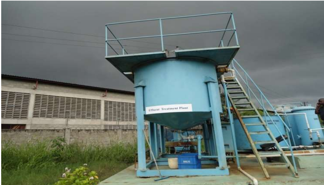
Plate 4.2: Wastewater treatment tank
