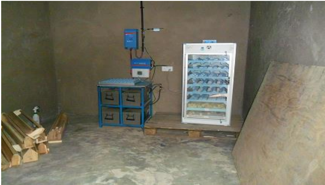
Figure 3.3: Inverter, Charge Control, Batteries with Monitor and Incubator
